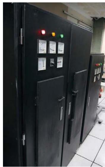
UPS (Uninterruptible Power Supply)
