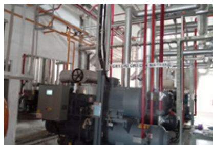
RUANGAN MESIN COLD ROOM
